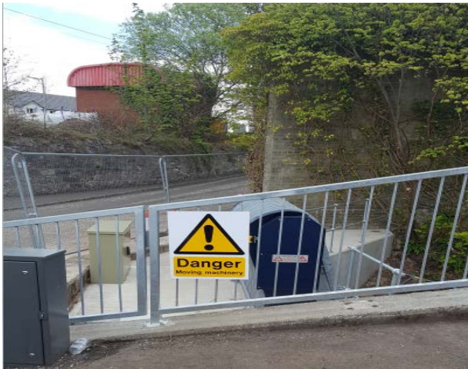
April 2017 at Installation– Left shows the top of the automated screen and control cabinet behind.
