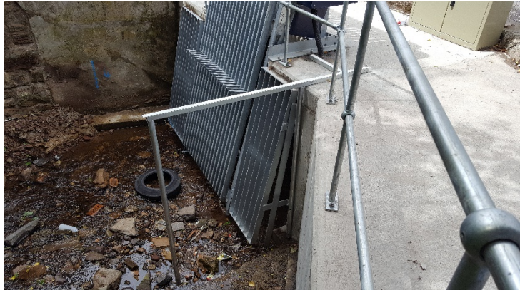
June 2017 after Installation – Below shows the level of the watercourse bed being below the automated screen.
